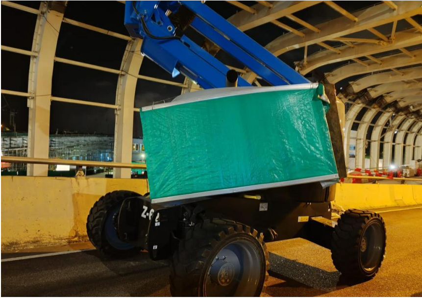
Remark 3: Acoustic shed and steel housing for cherry picker and mobile crane
